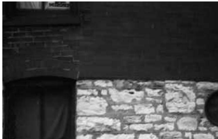
Figure 9a. An example of a deteriorating brick wall that has been tuckpointed, and a rock foundation.
