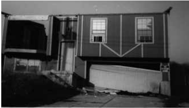
Figure 4b. Massive problems occurred in Green Jade Estates subdivision near St. Louis when homes were built on unstable ground.
