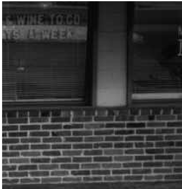
Figure 9c. Properly layed single brick wall.
