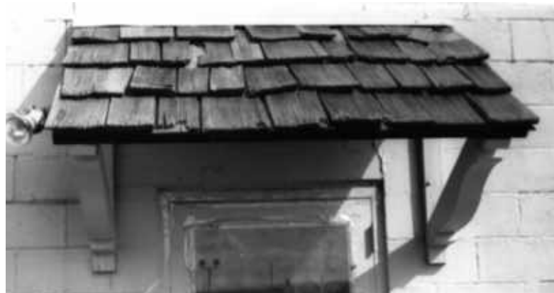
Figure 6. An example of deteriorating wood shingles.
