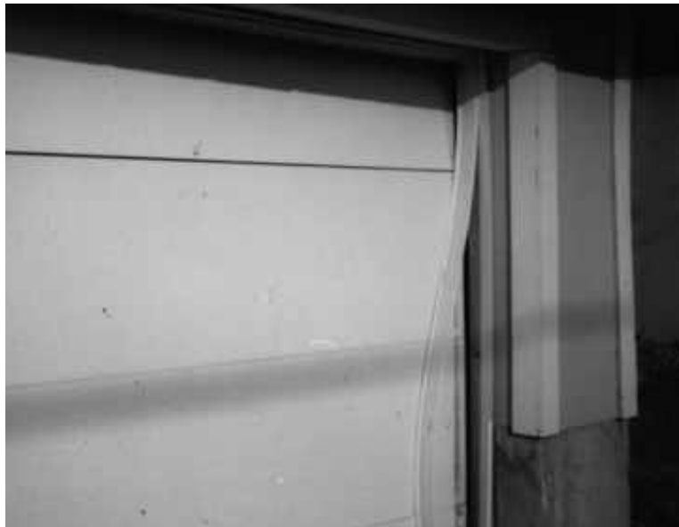
Figure 11b. Aluminum siding falling off this four-year-old house.
